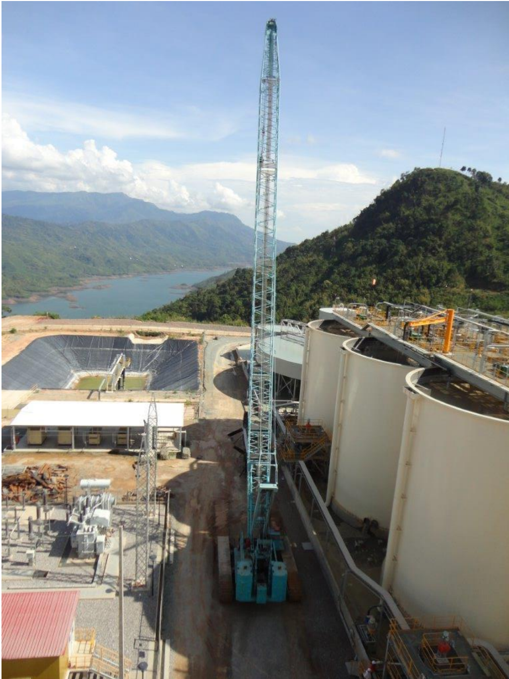
CIL plant with non-pumping screens. Shows cascade arrangement of tanks.
